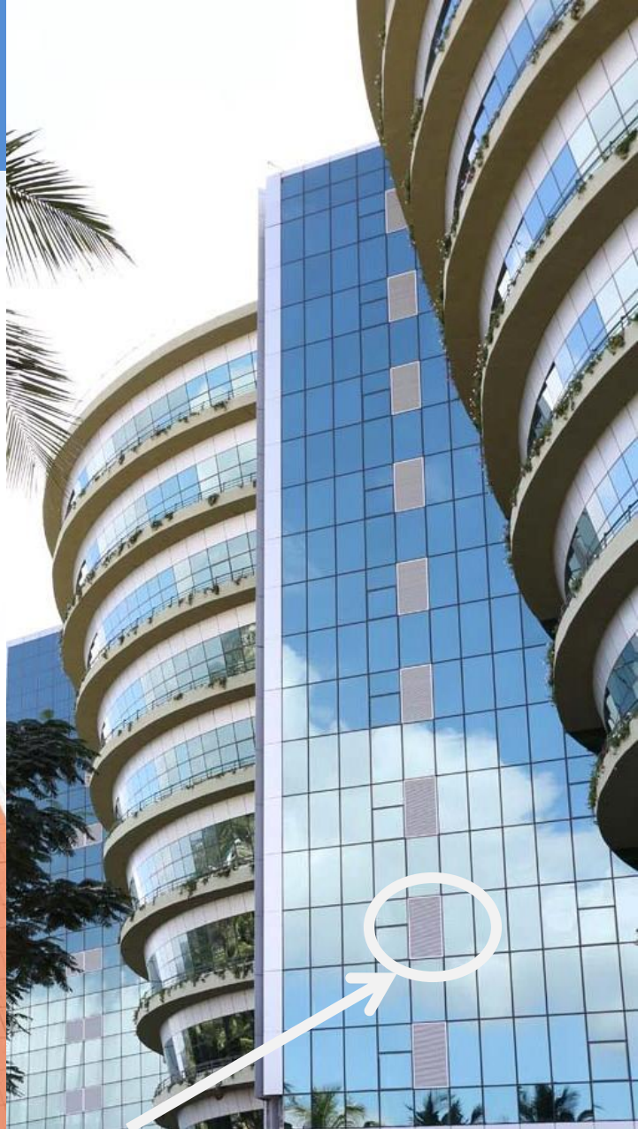
Exhaust grills with motorized dampers
